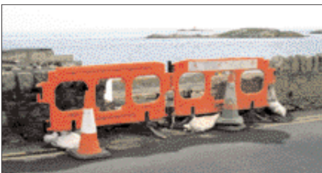
Left: Damaged wall at Coliemore
