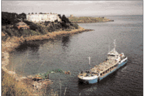
M B Jopi at work on coastal defences off Sorrento and The Vico, Dalkey Photo © Jehan Ashmore
